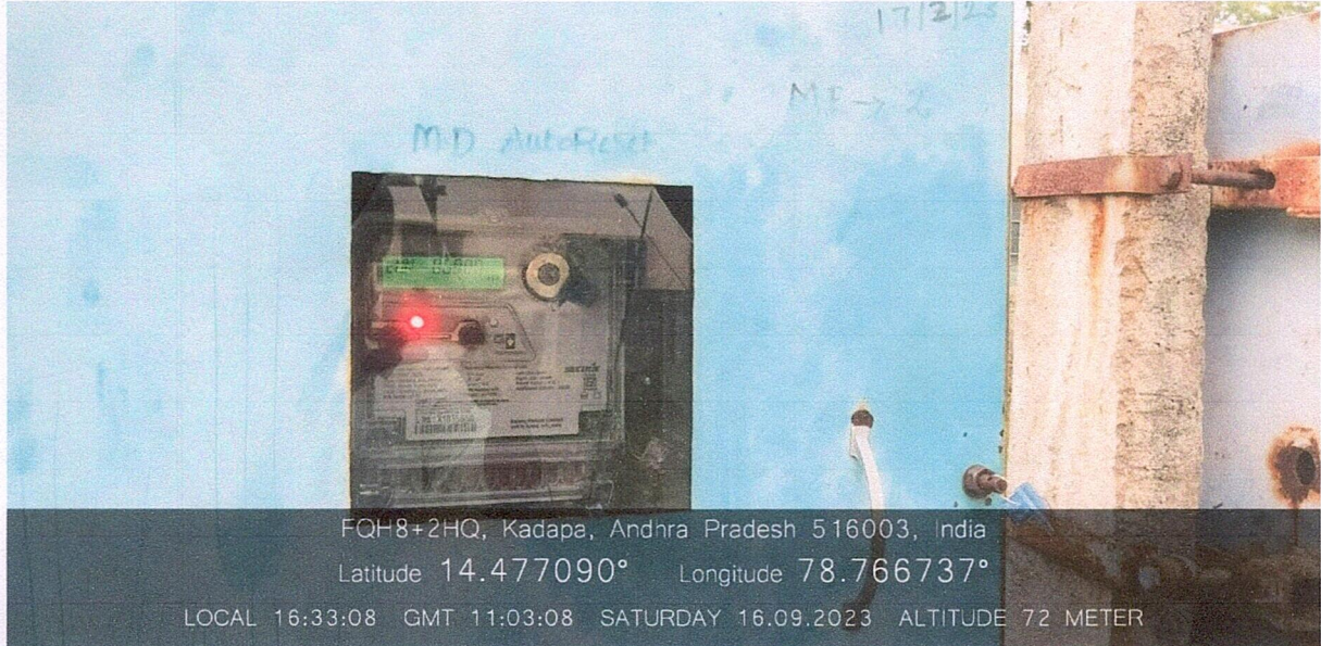
Wheeling to the Grid
