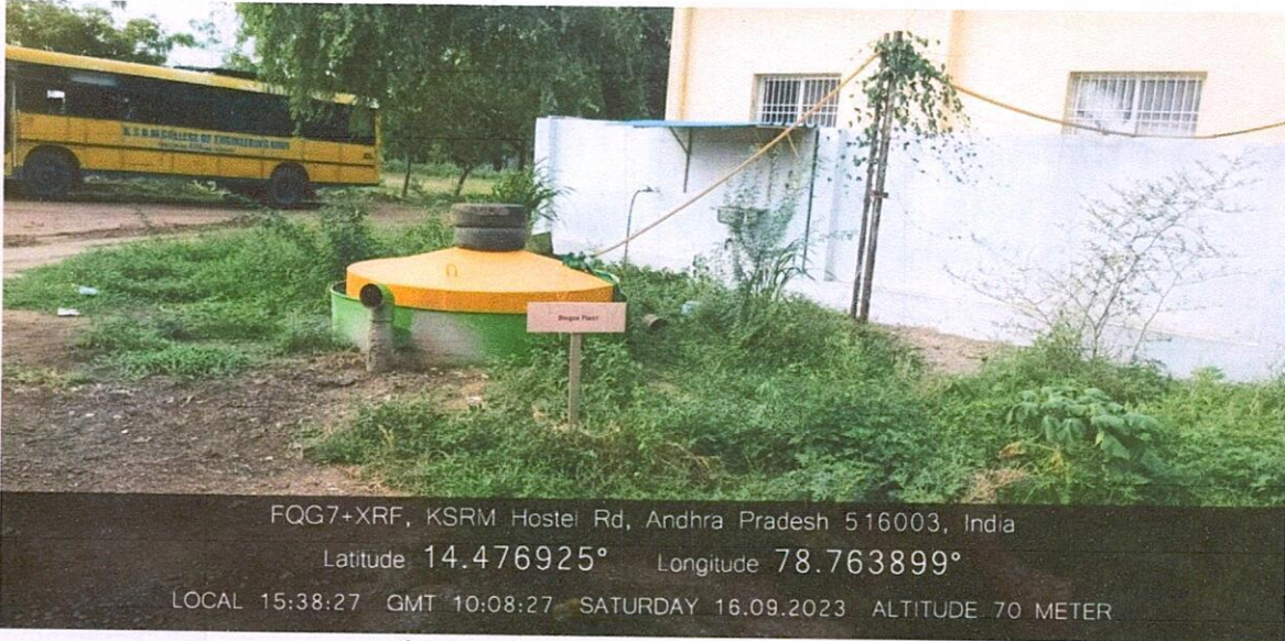
Biogas Plant near Central Kitchen
